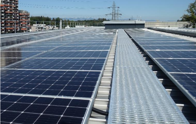
ROOFWALK Maintenance walkways between PV modules
